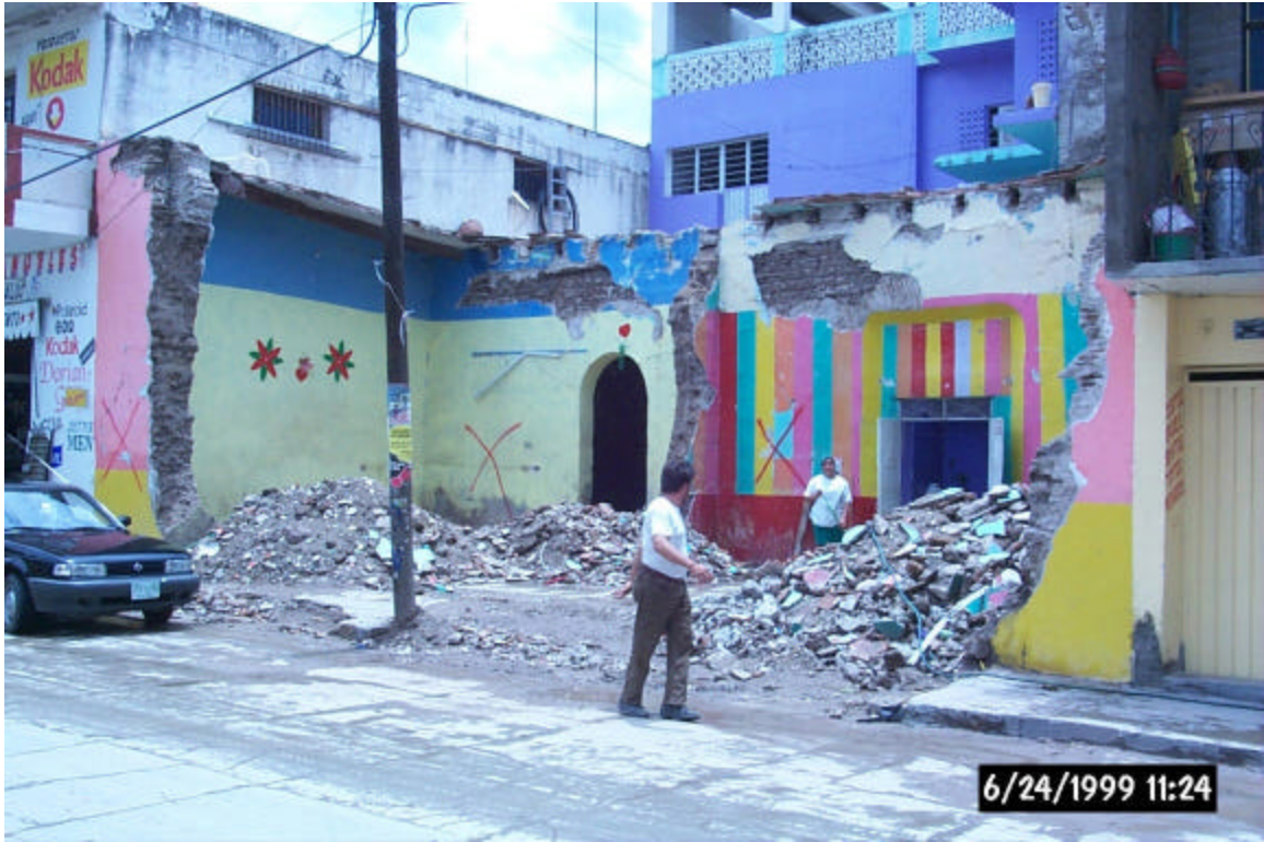
Figure 4.9 Demolished URM structure in Acatlán de Osorio.
