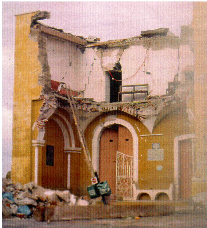
Figure 4.8 Damage to the Cholula church due in part, to topographic amplification of ground motions.
