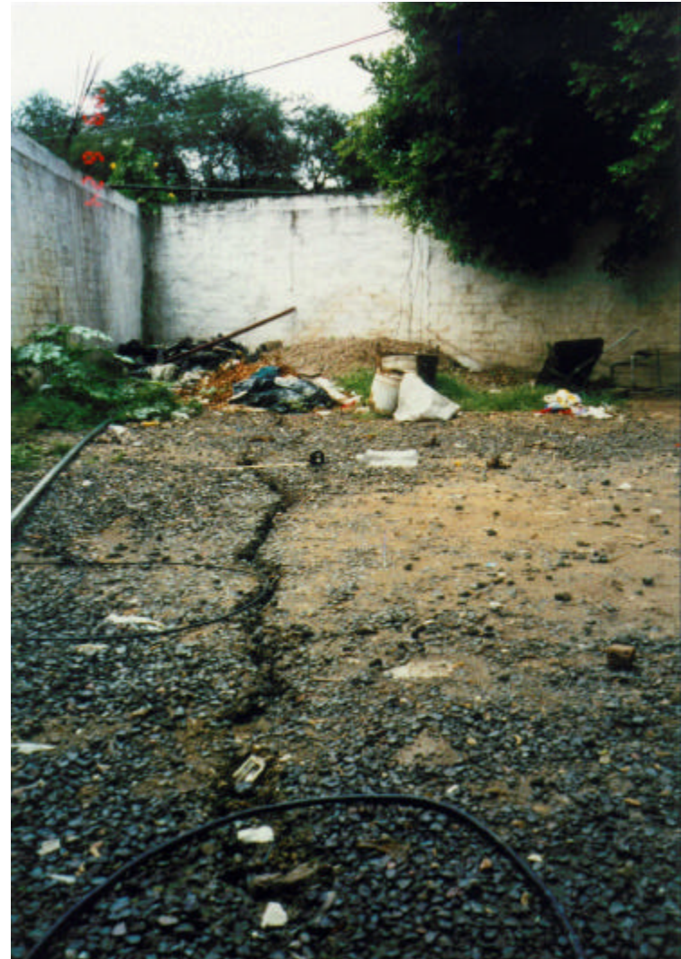
Figure 4.16 Lateral extension cracks in soil, Acatlán de Osorio.
