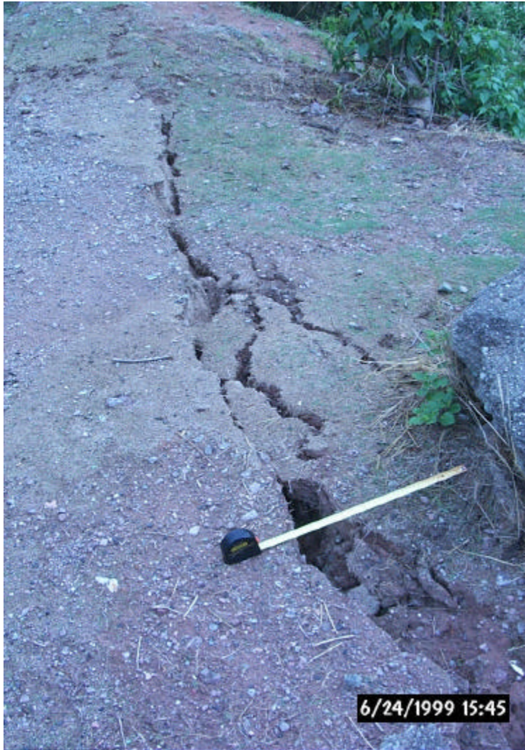
Figure 4.15 Slumping and cracking of soil near a steep slope adjacent to the highway at Puerto el Gato.
